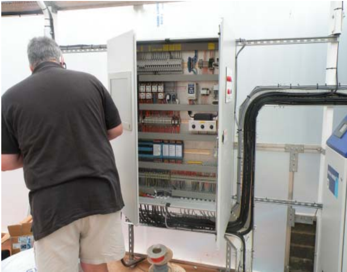
Electronics box with computer controller on the right
